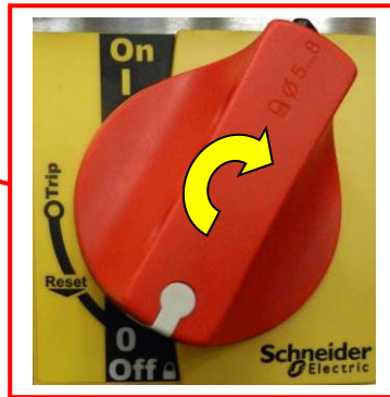
MAINS ELECTRICAL ISOLATOR SWITCH
