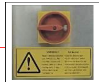
MAINS SUPPLY ISOLATOR
