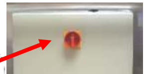
PROVER MAIN ISOLATOR
